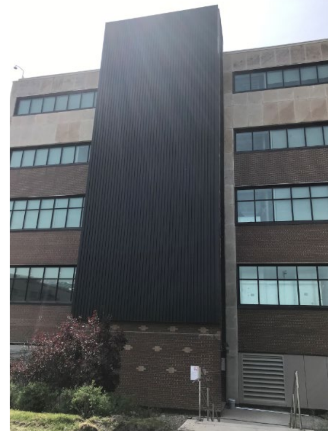
Solar wall installed at one of our Head Office buildings in Ottawa.
